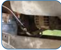
Leak from low pressure connection.
